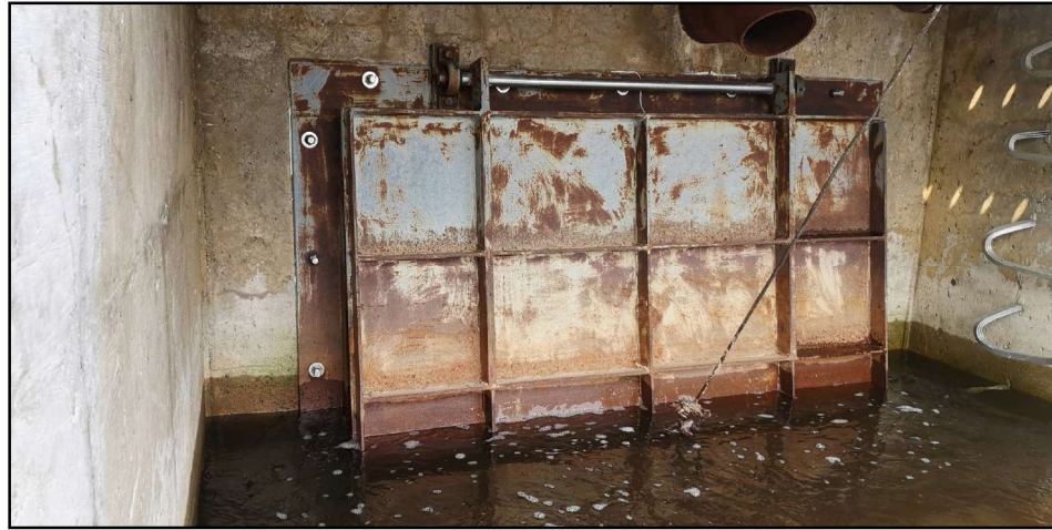
Figure 5 OMC Outlet Flap Gate
