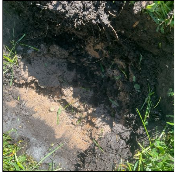
Image 6: Example of disturbed Test Pit conditions. Note lack of topsoil.
