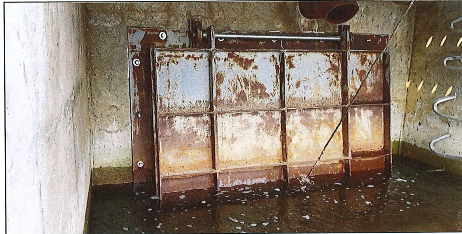
Figure 5 OMC Outlet Flap Gate
