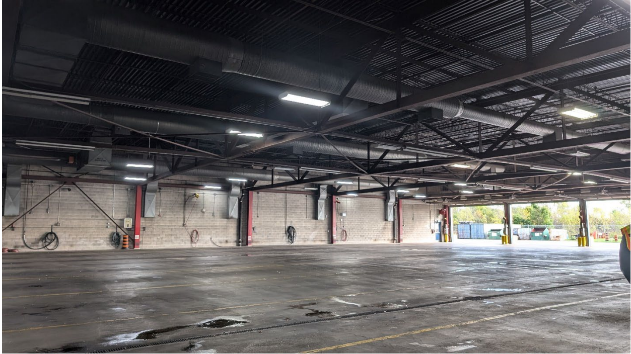
Figure 2-5: Ducting in Original Bus Storage Area.
